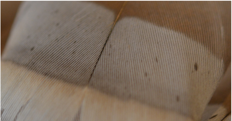
Fig. 210: Black leakage in the slated areas
